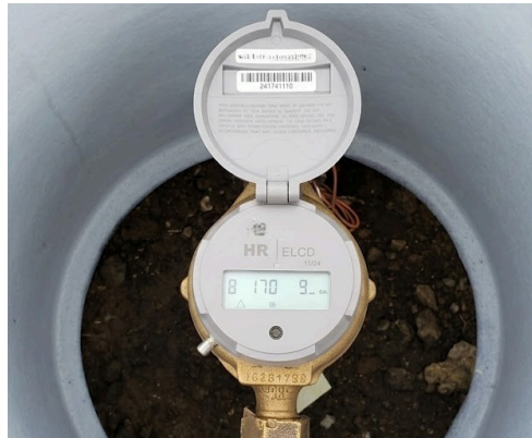
Advanced Metering Infrastructure (AMI)
